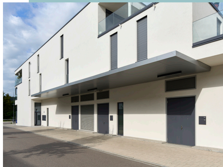
External steel doors to the commercial units. The robust steel elements blend in visually with the overall appearance of the complex and protect against break-ins with security class RC3.
