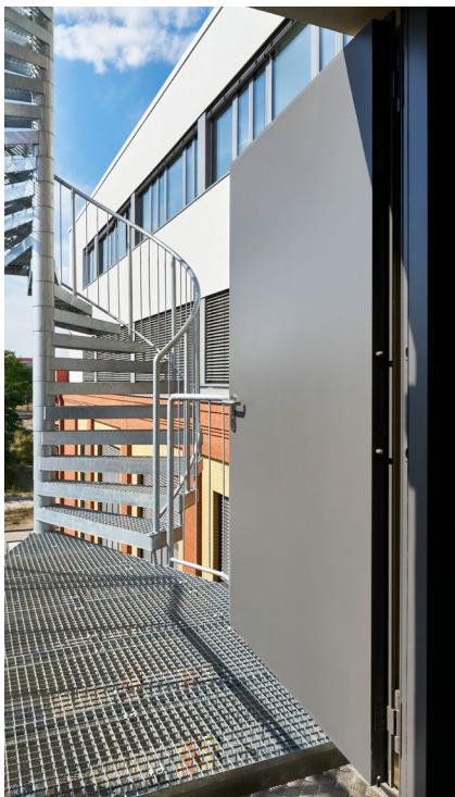
Stair tower with escape doors. The security doors are equipped with special block frames.
