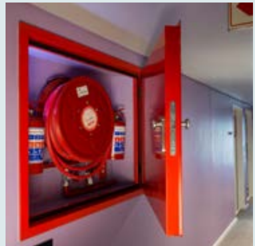
Fire-protection hatch in Radisson Red.
